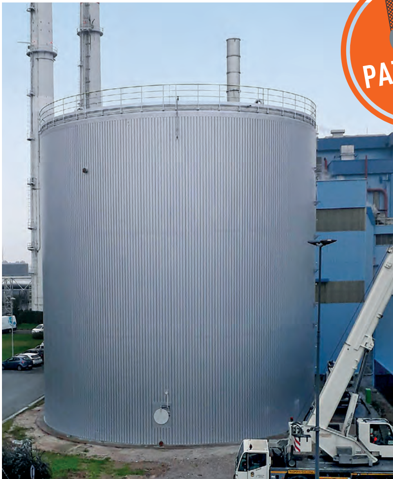
LIPP Thermal Storage Tank, 5,200 m 3 volume
