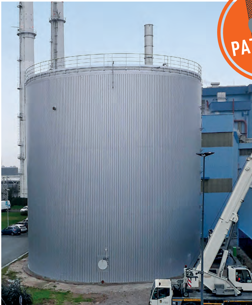
LIPP Thermal Storage Tank, 5,200 m 3 volume
