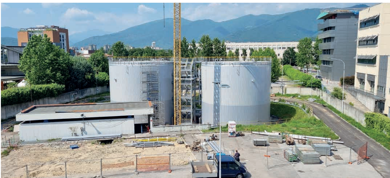
Figure 4. Lipp welding technology was used to construct two thermal storage tanks at the Centrale Nord power plant site
