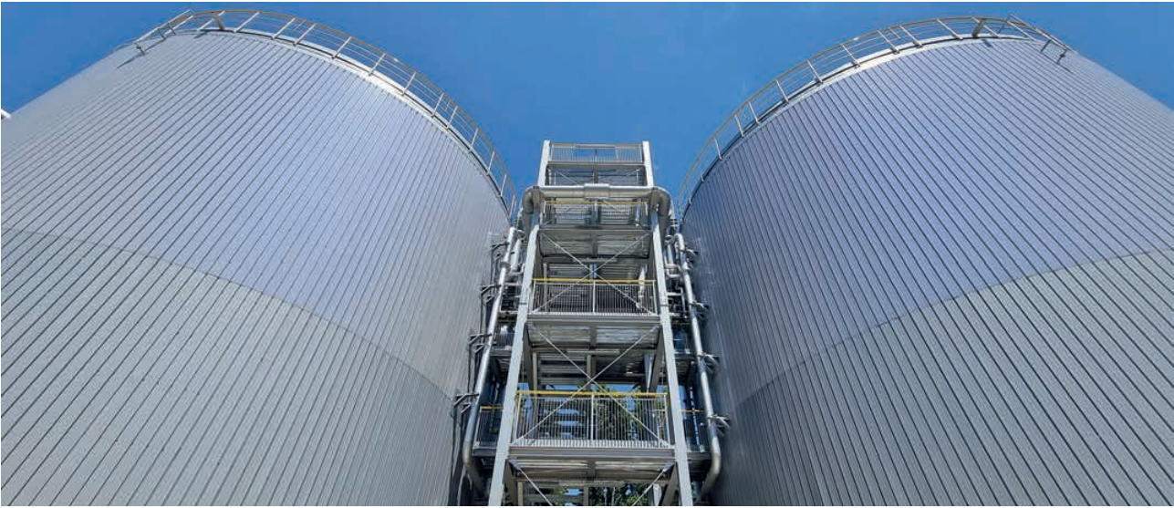
Two thermal storage tanks, each with a capacity of 2,200 m 3 , have been built at the Centrale Nord power plant site in Brescia, Italy
